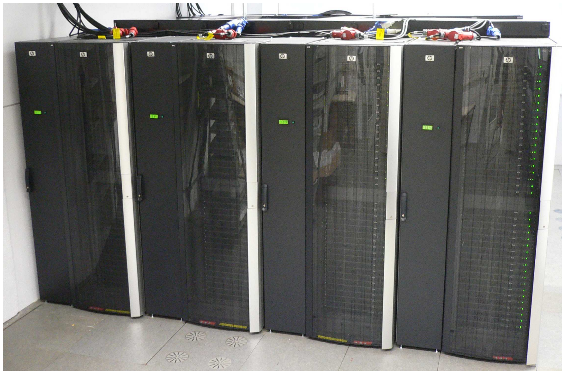
One row of water cooled racks
